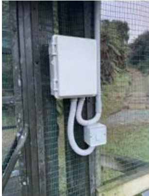
New pin pad entry at Lee Bay
